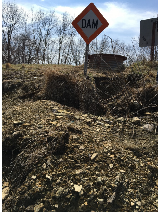
Photograph 5 upstream damaged embankment
