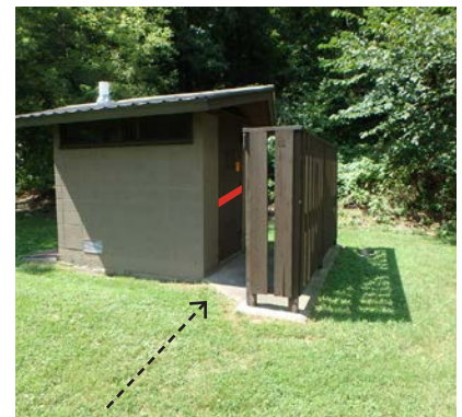
High-Level Deficiency Add accessible route (on steep slope) and modify entrance threshold.
