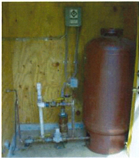
Pressure tank, Switch
