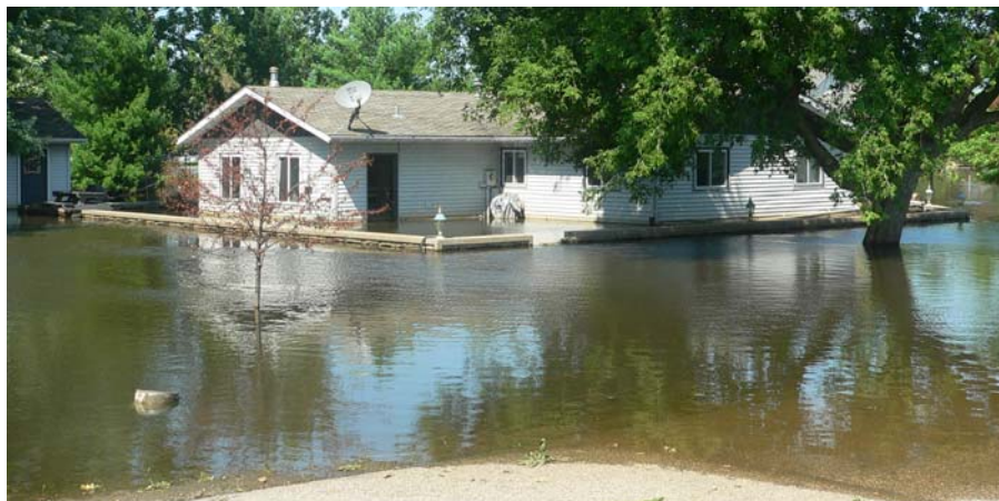
Figure 1.5-1. Failure of Post 1993 Installed Flood Protection in the Prairie View Subdivision Source: Jewell Associates – Taken July 2008.
