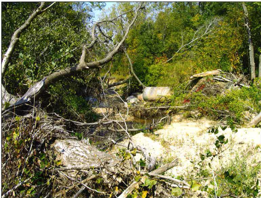
Debris pile and erosion in middle reach of Clark Creek.
