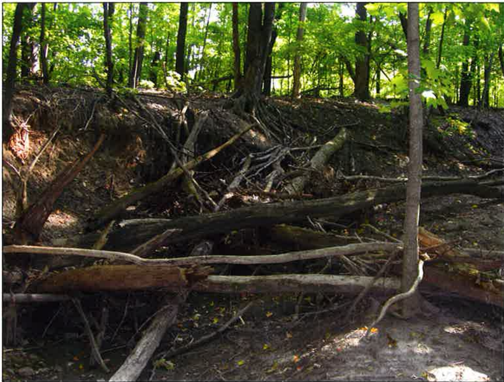
Debris pile in the channel of an intermittent reach of Clark Creek near Tower Road.
