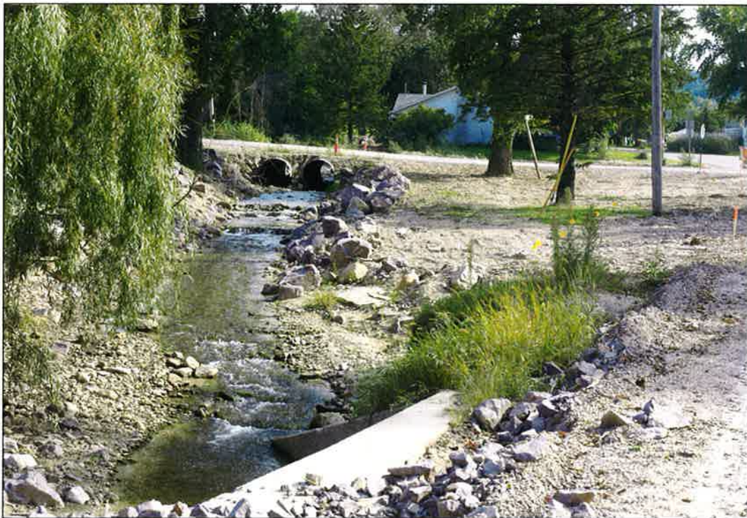
Misaligned Highway 113 box culvert in foreground and County Road W dual corrugated metal pipe culverts in background in lower reach of Clark Creek.
