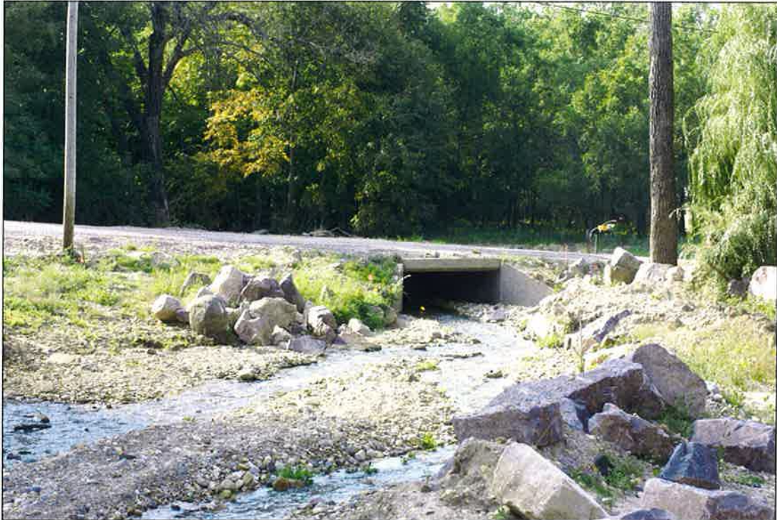
Misaligned Highway 113 box culvert near Maxwell Farm at downstream extent of rechannelization of Clark Creek.
