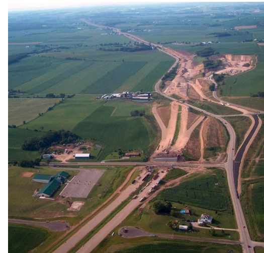
Construction between Sauk City and Middleton during the first phase of the Highway 12 improvements.
